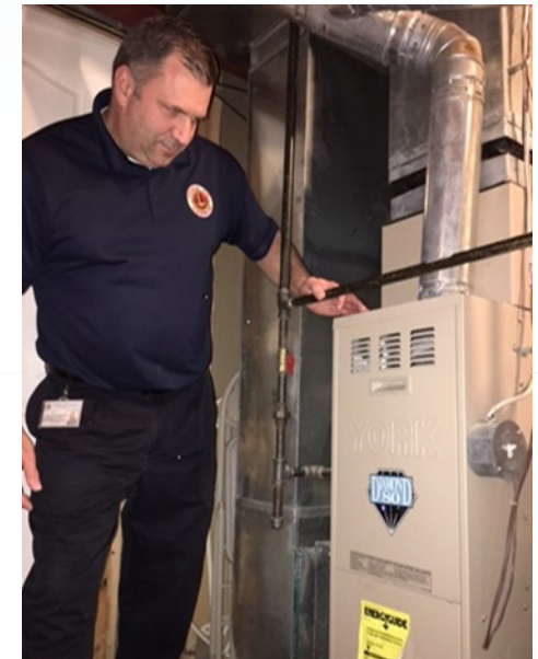
A GRIP Building Inspector verifying the installation of an applicant's new furnace.
